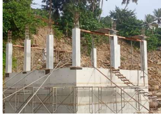
Underground water sump
